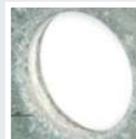
16months (Zinc Magnesium) 10% red rust 70% white rust
